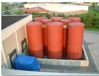
Cutting / Cooling Oil Mixing Plant
